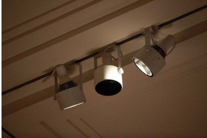
Figure 4. Track luminaires installed in the gallery with Cree 12W PAR38 LED replacement lamps.
